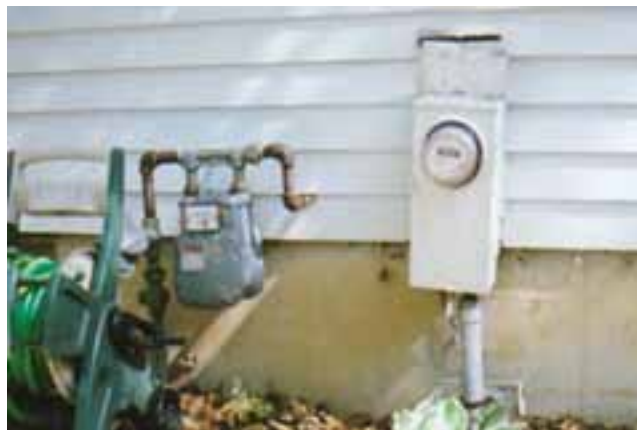
Figure 5.4: An electrical service box torn from a home because of soil settling.
