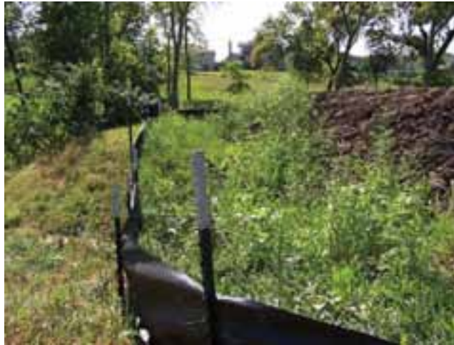
Figure 3.10: Silt fences collect sediment and keep it from reaching water bodies near construction sites. Construction is just starting on this site.
