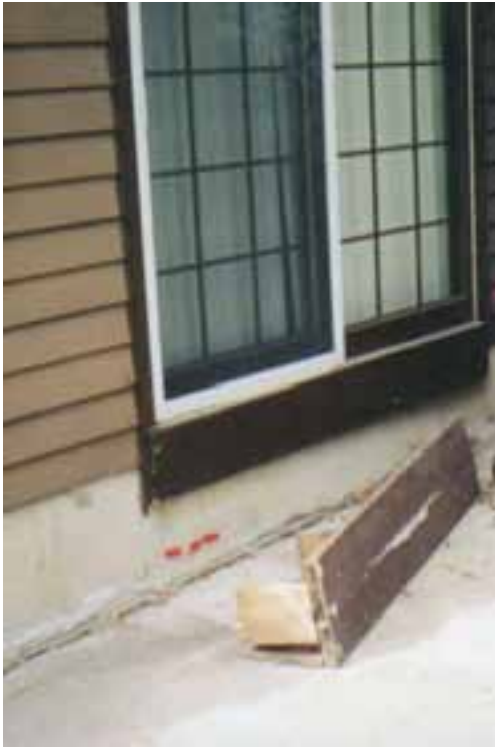
Figure 5.5: A home damaged by soil settling.
