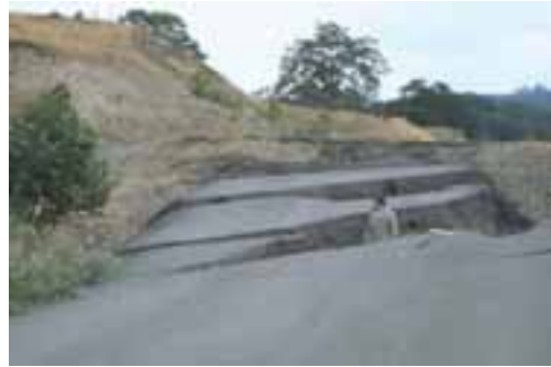
Figure 5.6: A road constructed on an unstable soil.
